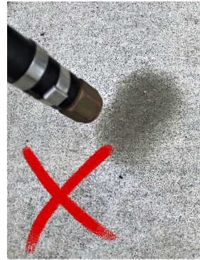
Figure 6 Moisture and Discoloration Present
