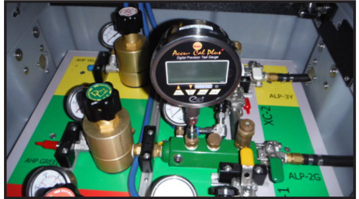
Figure 8. HP Gauge Installed for XLDS Low Pressure Gauge Comparison
