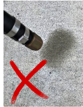
Figure 6 Moisture and Discoloration Present
